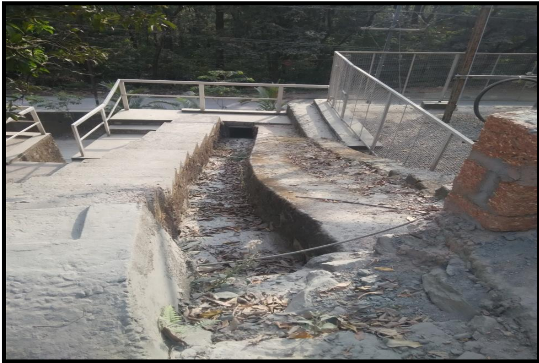
Garland drains for storm water management
