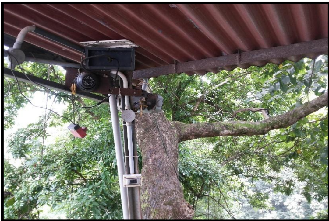
Warning alarm installed in the project site
