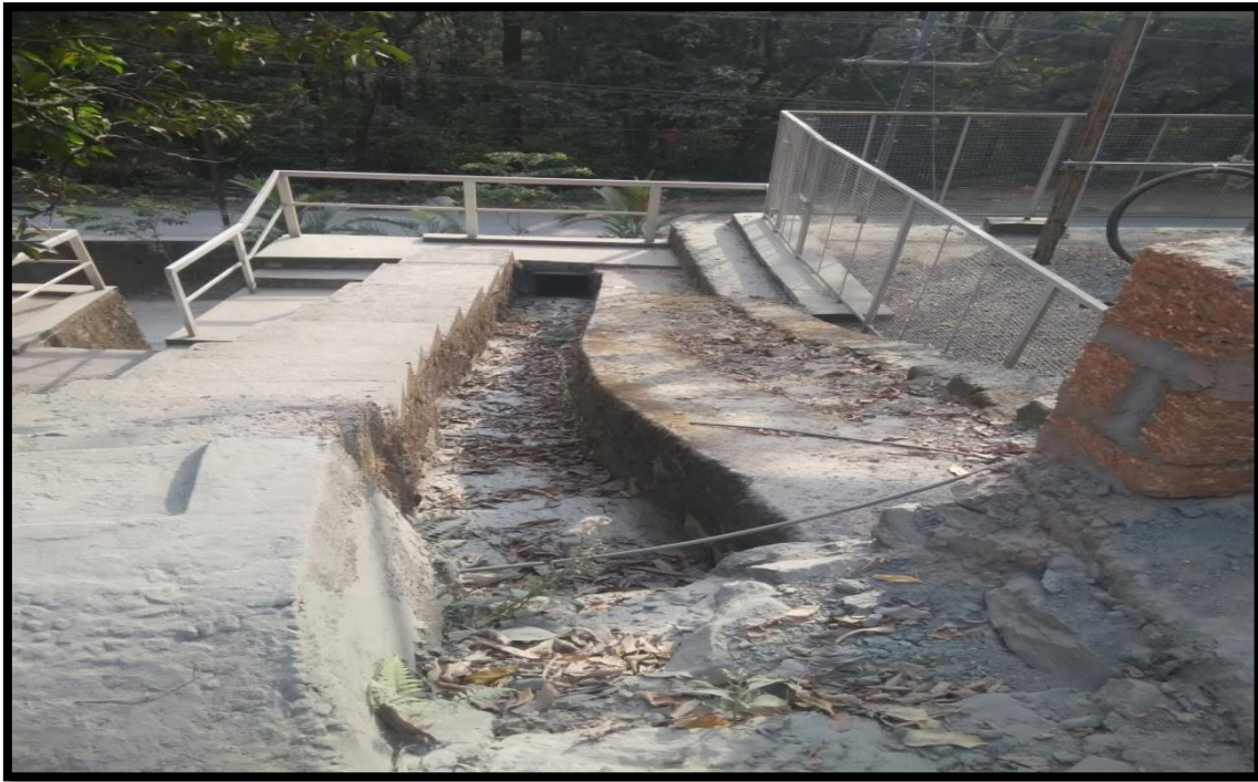
Garland drains for storm water management
