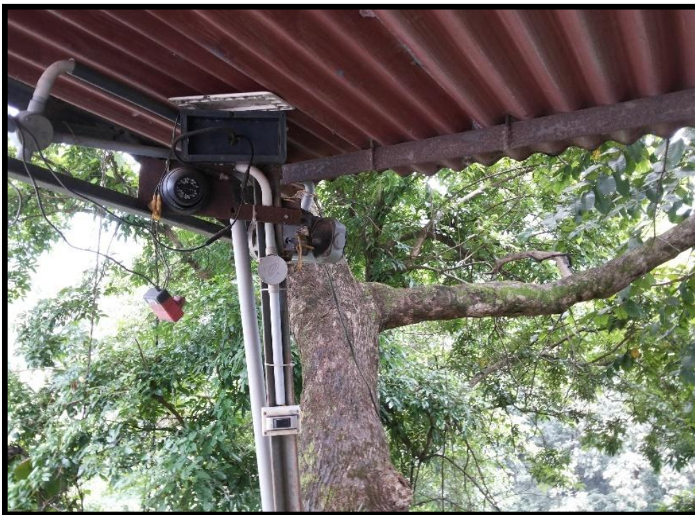
Warning alarm installed in the project site
