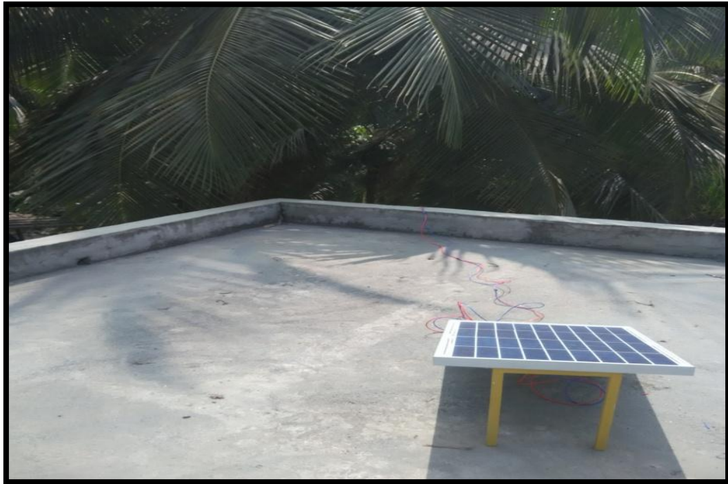
Solar panel installed in project site
