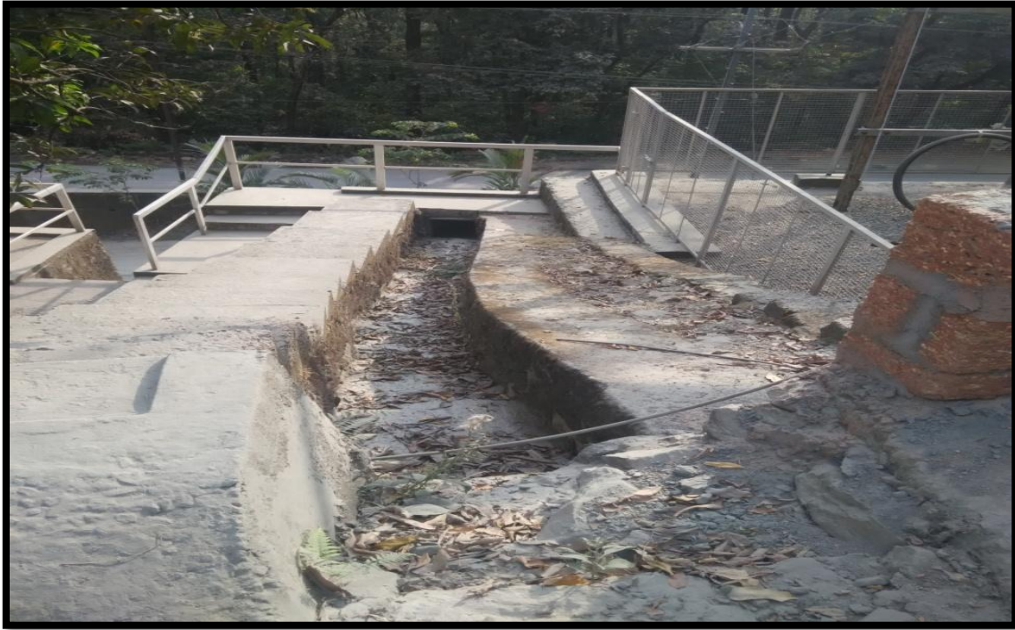
Garland drains for storm water management
