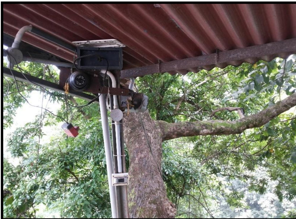
Warning alarm installed in the project site
