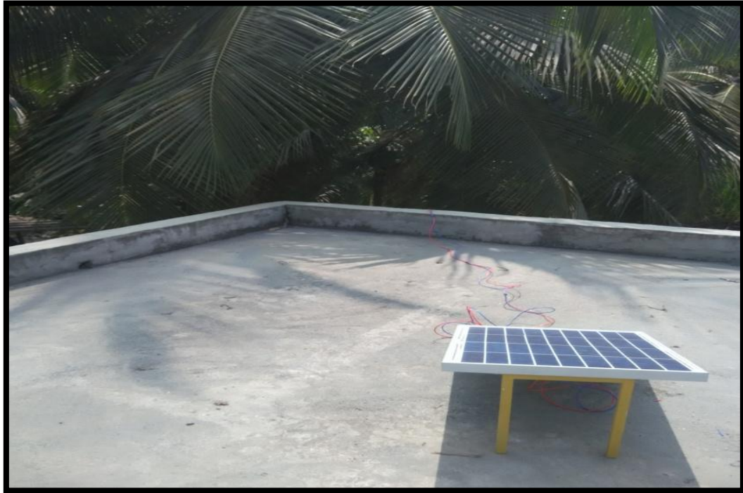
Solar panel installed in project site
